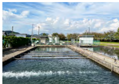
Drainage treatment facility in Takefu Plant
