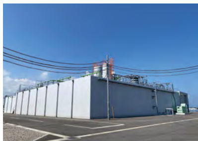
Wastewater treatment facility in Oita Plant
