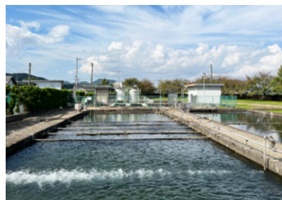
Drainage treatment facility in Takefu Plant
