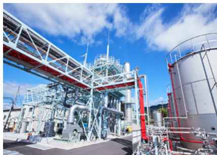
Submerged combustion system at Yanai headquarters plant (newly installed)
