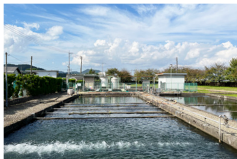
Drainage treatment facility in Takefu Plant
